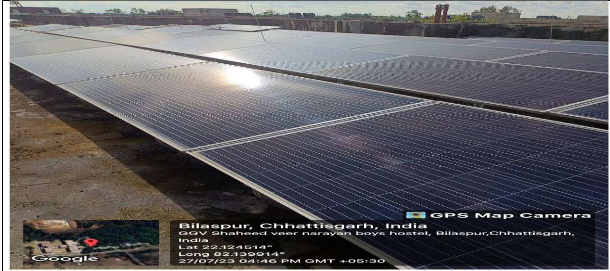
Roof Top Solar Panel – Boys Hostel
