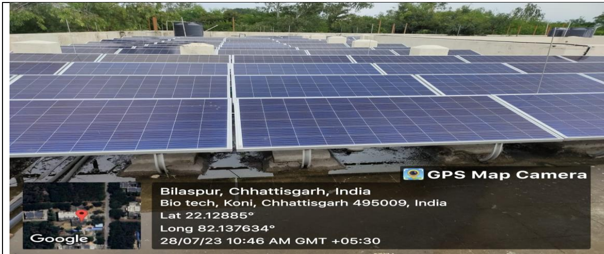
Roof Top Solar Panel – Bio-tech Department
