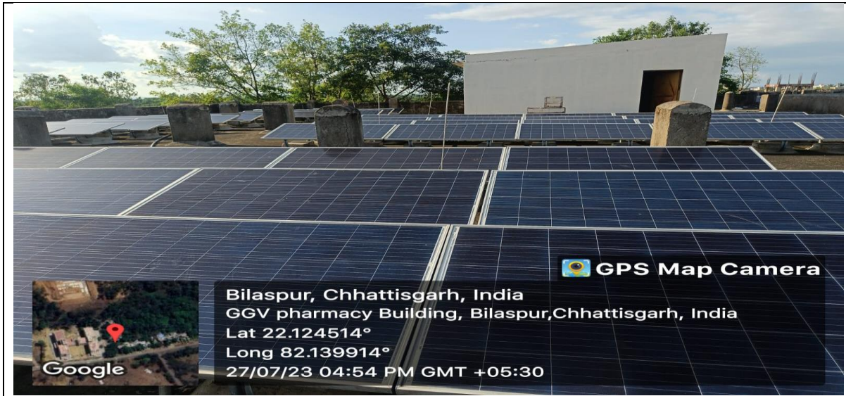
Roof Top Solar Panel – Department of Pharmacy
