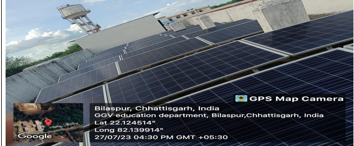
Roof Top Solar Panel – Education Department
