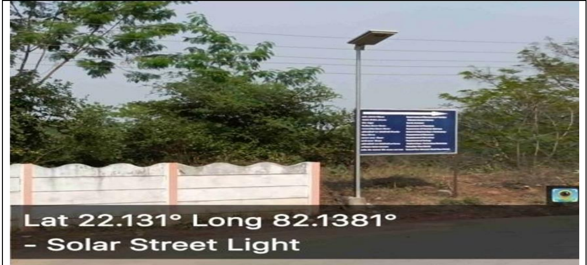
Sensor based Solar Street Light – Near Pond
