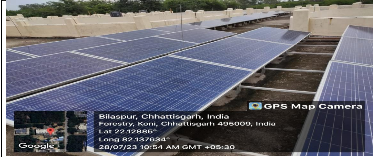
Roof Top Solar Panel – Forestry Department
