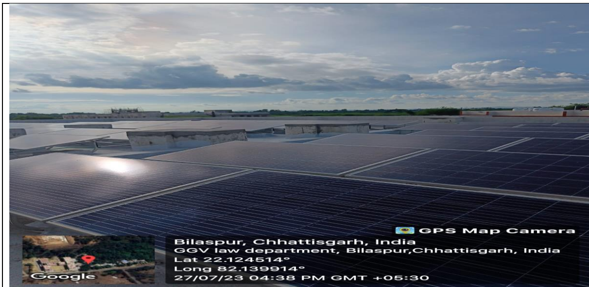
Roof Top Solar Panel – Department of Law
