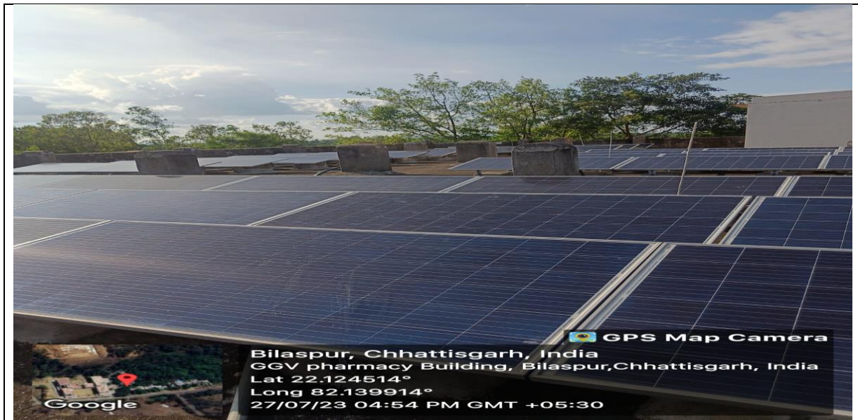
Roof Top Solar Panel – Department of Pharmacy
