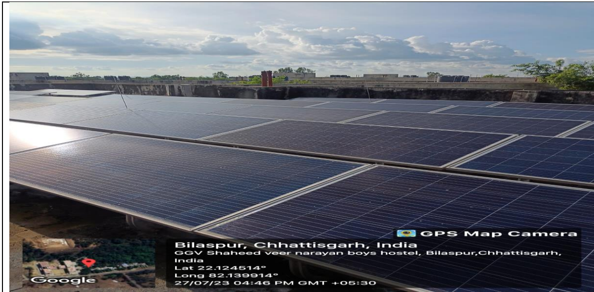
Roof Top Solar Panel – Boys Hostel
