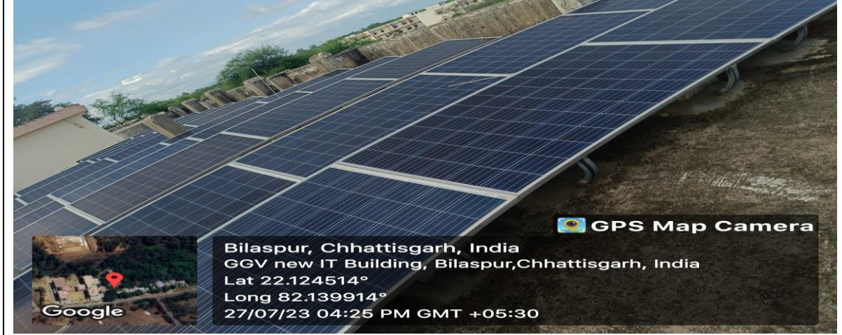
Roof Top Solar Panel – New IT building
