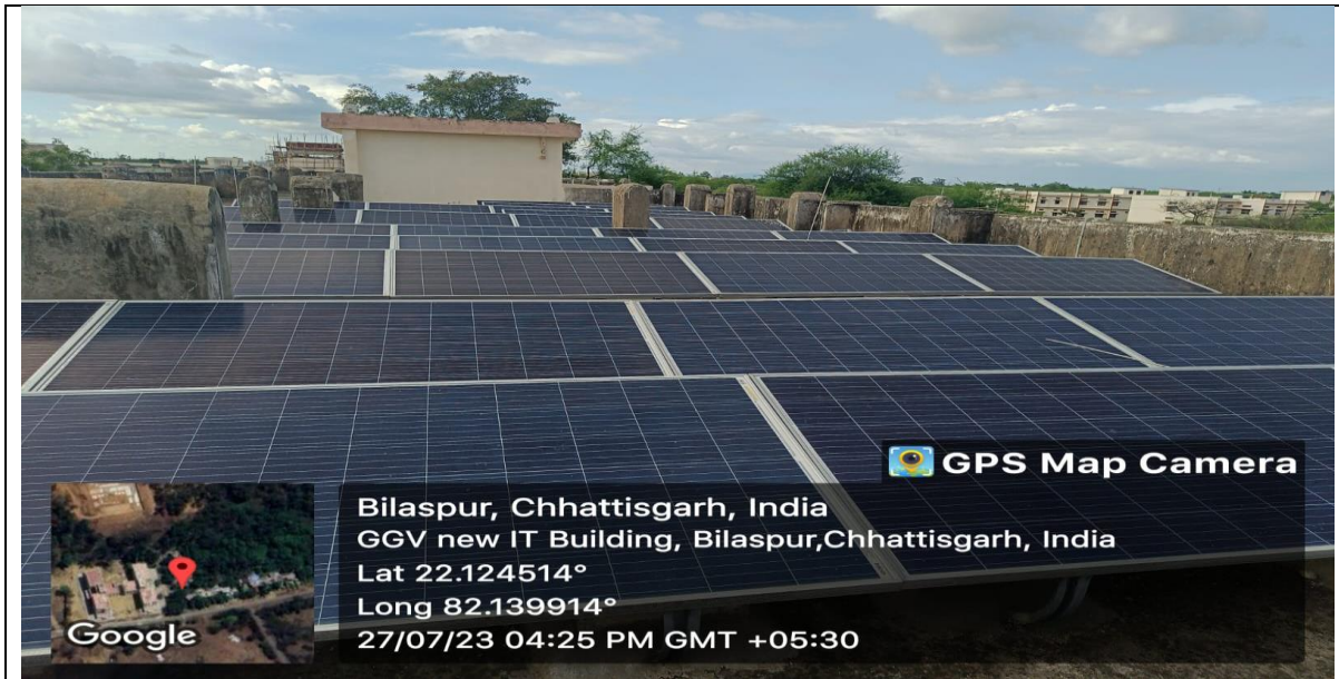
Roof Top Solar Panel – New IT building
