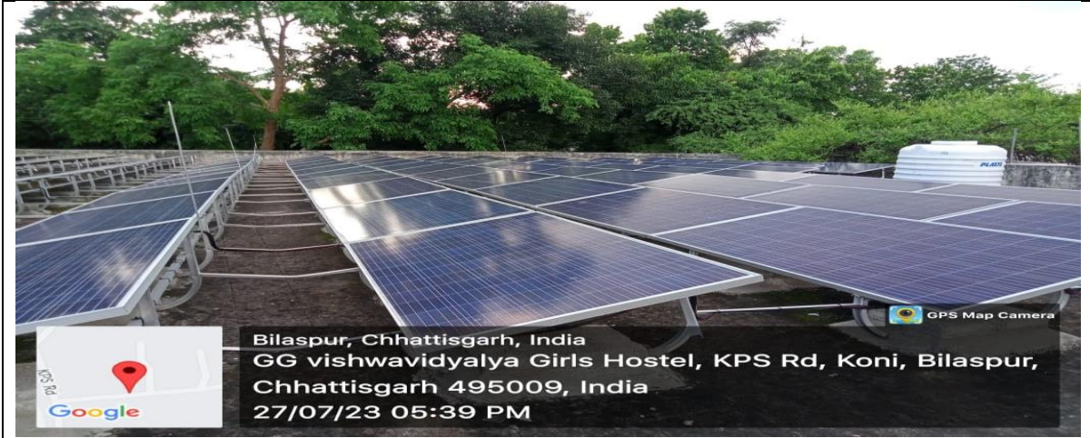
Roof Top Solar Panel – Girls Hostel
