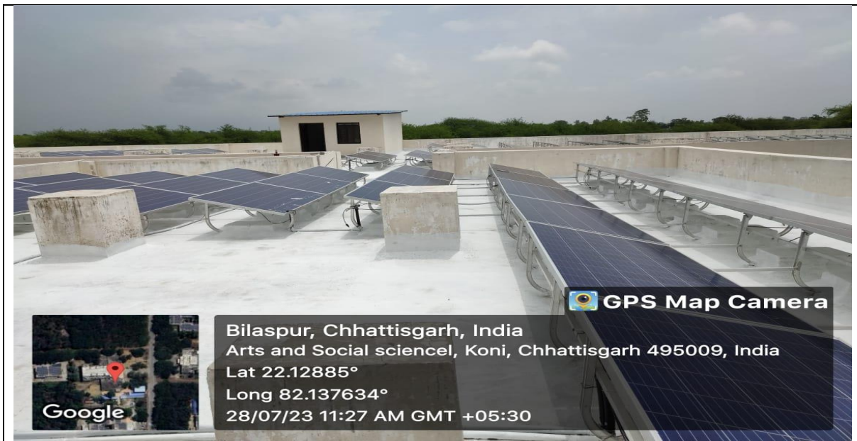
Roof Top Solar Panel – Arts and Social Science
