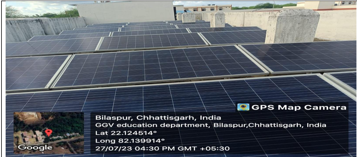
Roof Top Solar Panel – Education Department
