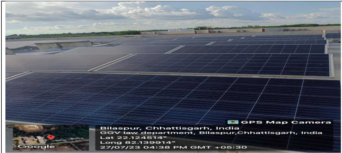
Roof Top Solar Panel – Department of Law
