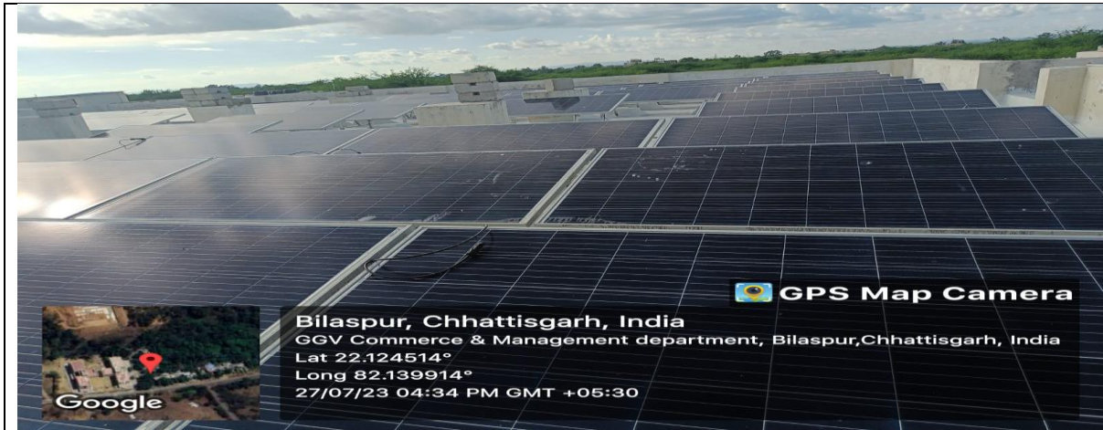
Roof Top Solar Panel – Commerce and Management
