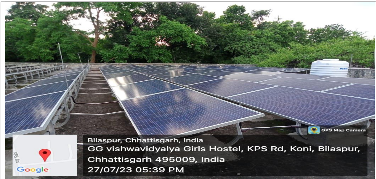
Roof Top Solar Panel – Girls Hostel
